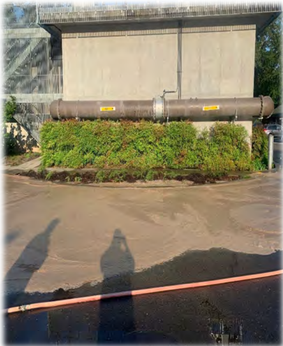
Digester 3 Foam Over.
