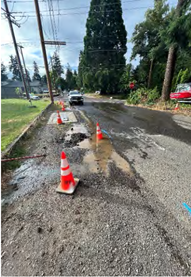
Main break on Addie St at Jennings Ave.
