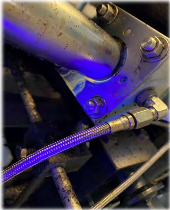
Florescent Dye Used to Identify Hydraulic Leak.
