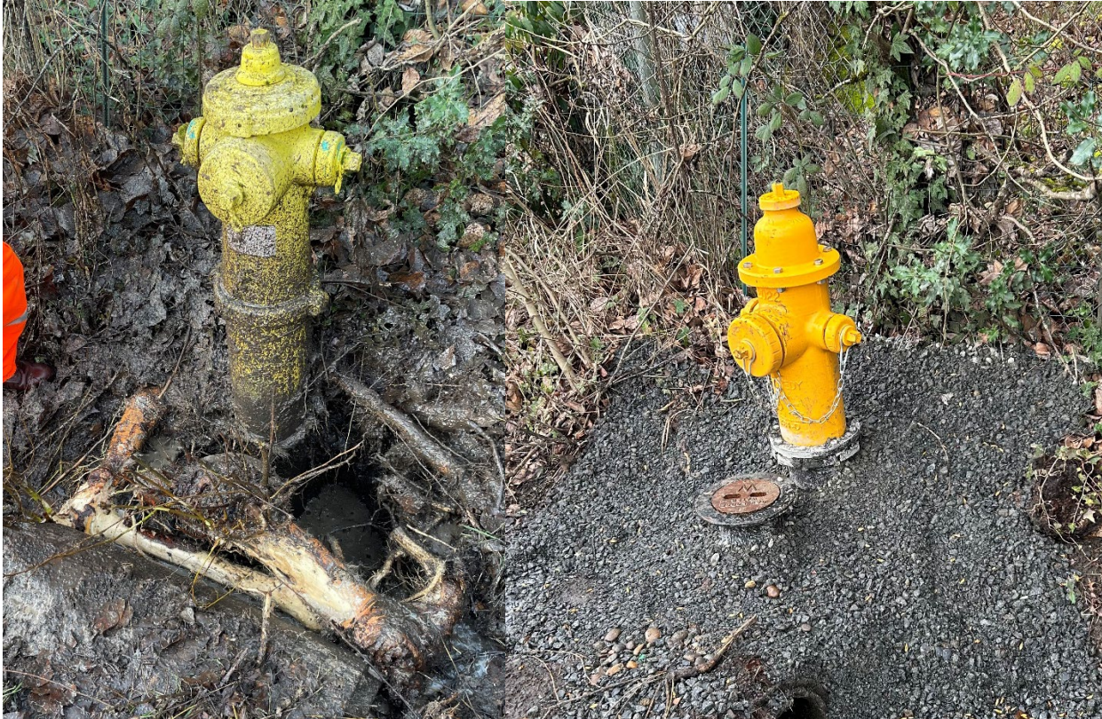
Existing Boardman Hydrant
