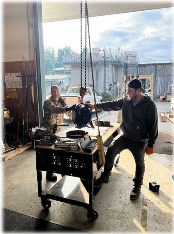
Maintenance rebuilding a rotary Lobe pump.
