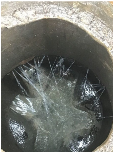
MH I&I Before
