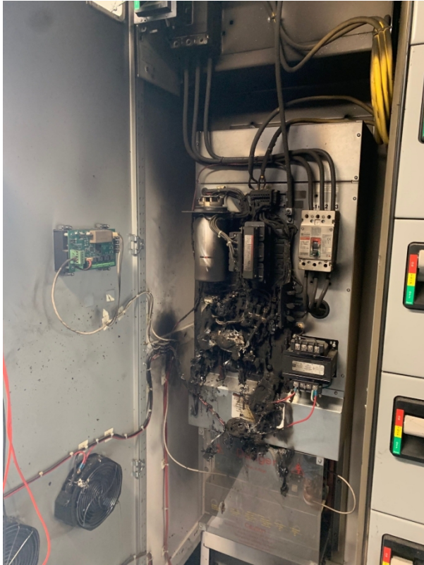
Harmonic Correction Unit that caught fire.
