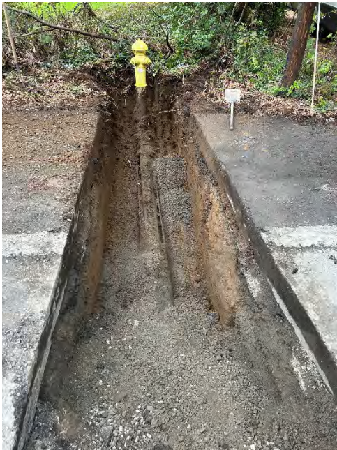
Old 2 port hydrant River Rd
