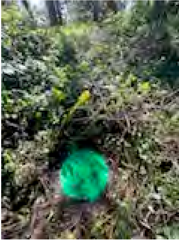
Missing manhole structure located
