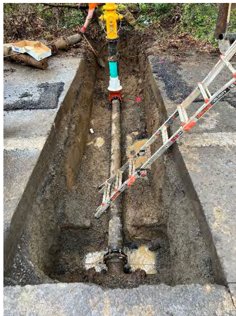
New 3 port hydrant on River Rd
