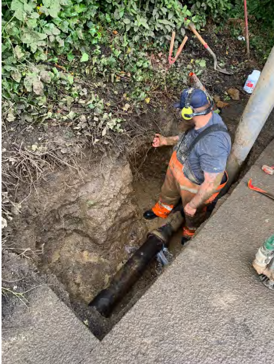
(1) Picture of main leak on the South side of Jennings Avenue, West of Oatfield Road.
