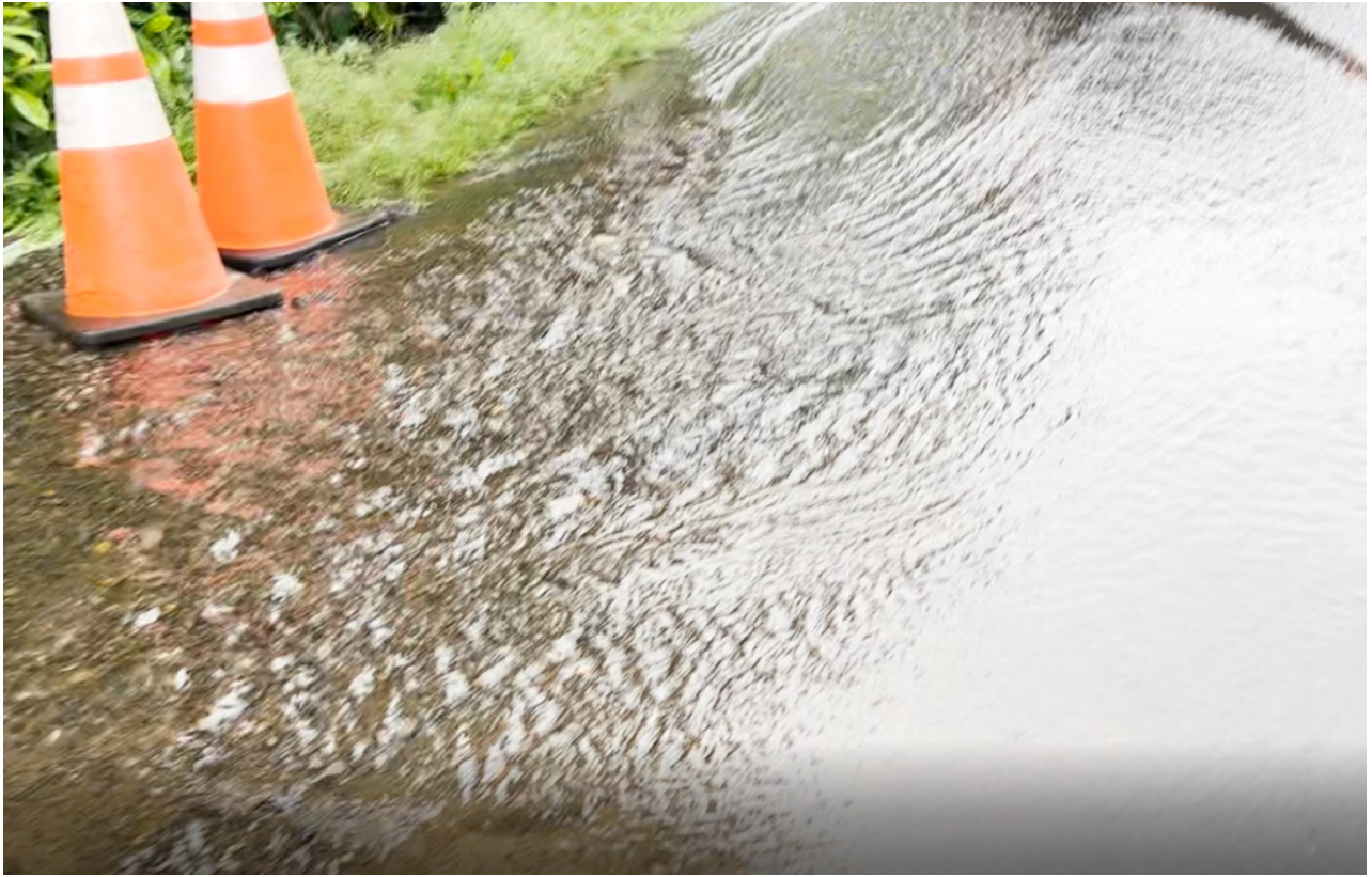
Photo 5: Main leak in front of 14522 SE River Road
