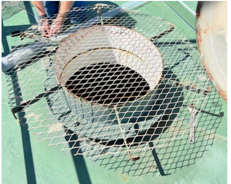
Photo 2: Finer vent screening needed for smaller debris
