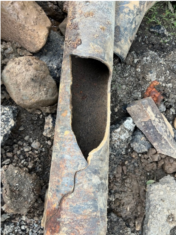
Photo 6: Broken pipe removed from River Road leak
