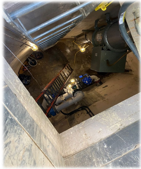
Inside the newly improved Lift Station 5
