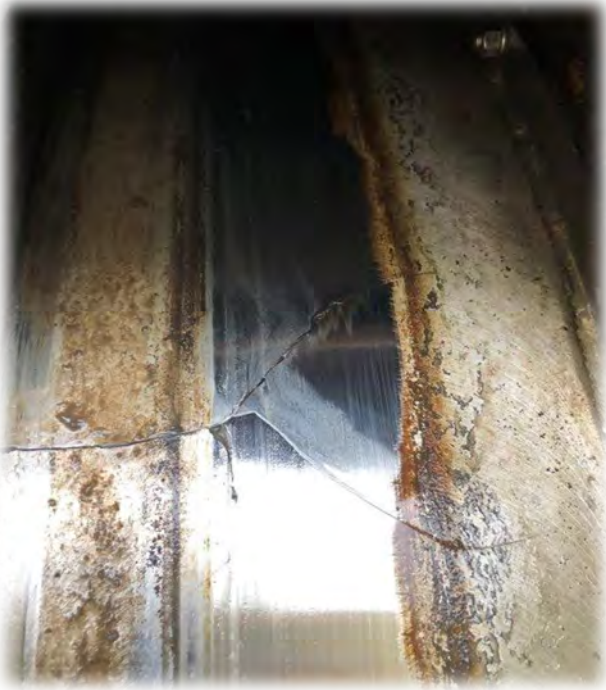
(5) Drum Screen Crack
