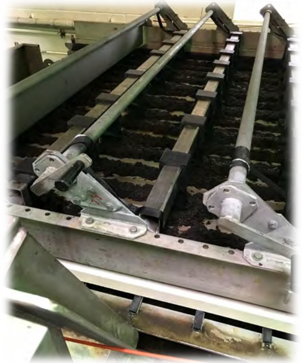
2) Belt Filter Press at Salmon Creek
