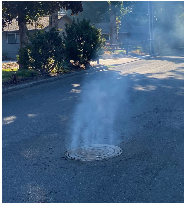
Photo 2: Smoke venting from manhole (normal)
