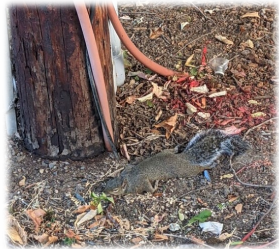
4. Prime suspect in the pump station 5 power loss.
