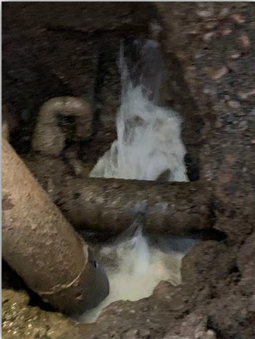
Water main was full circle break.
