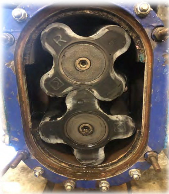
3) Digested Sludge Pump lobes
