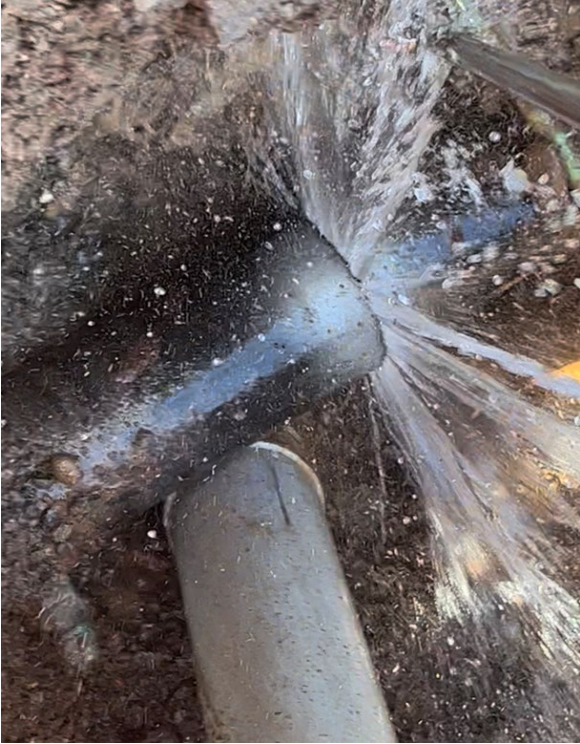
Photo 6: Radial crack on 6-inch cast-iron main on Oatfield Road
