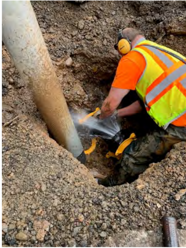
(1) Picture of main leak on Oatfield Road North of Jennings Avenue.
