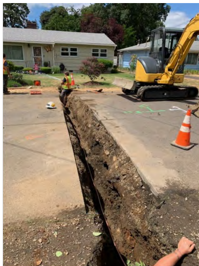
(3) This picture shows the crew renewing a plastic long side water service.
