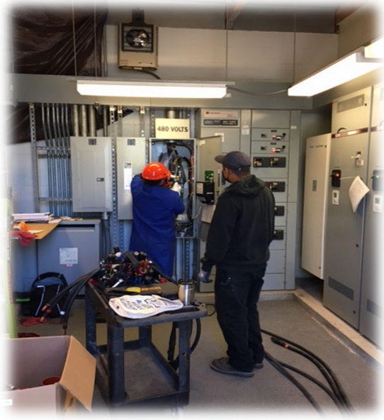
6) Pump Station # Generator Service
