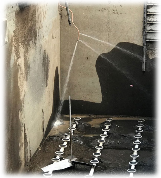
2) AB#1 showing broken mixer shaft
