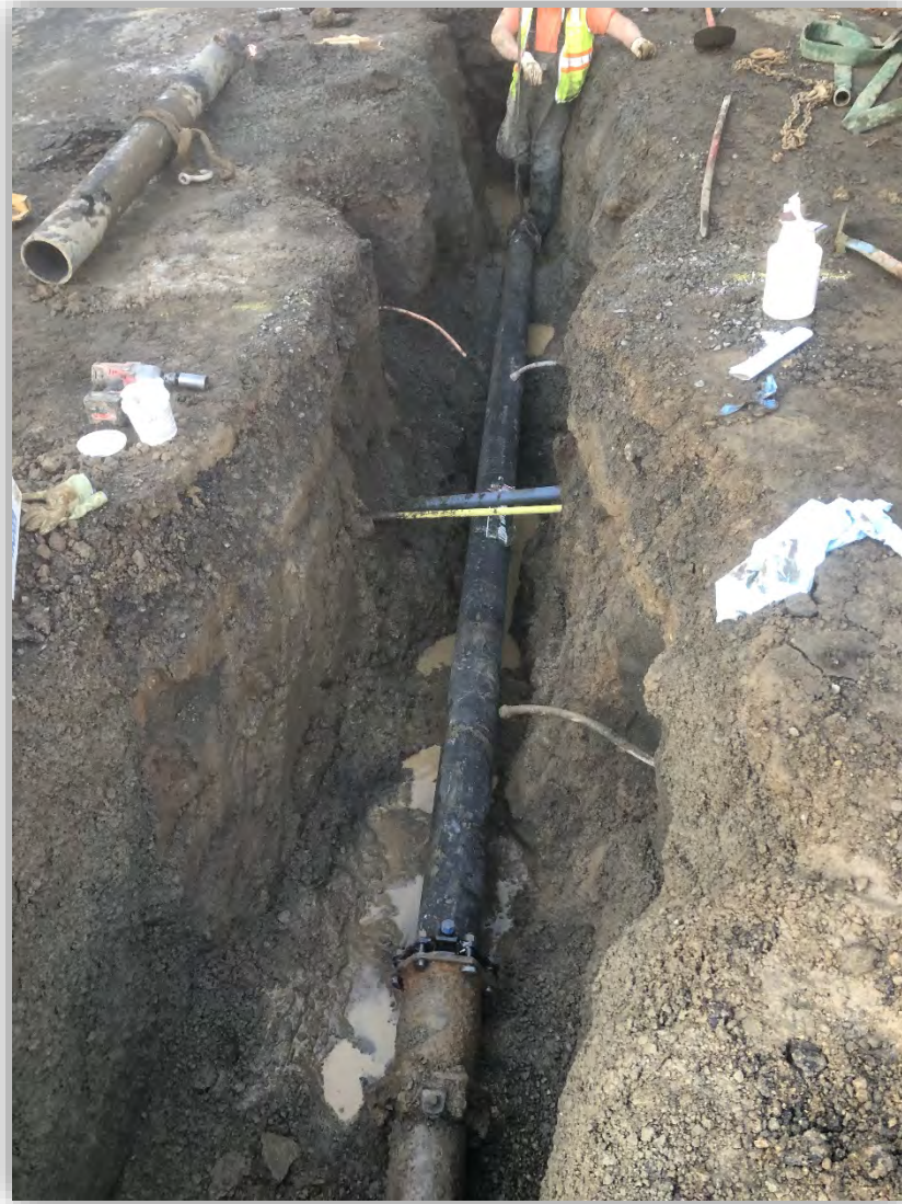
Main Break Colina Vista (11/8/20)
