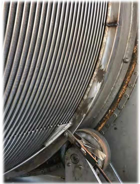
Drum Screen Welds
