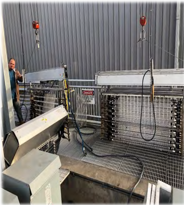
UV Equipment Cleaning
