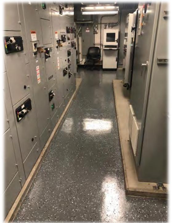
Building 15 Motor Control Center
