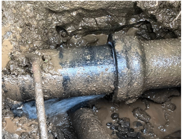
Photo 8: Exposed leaking bell-joint
