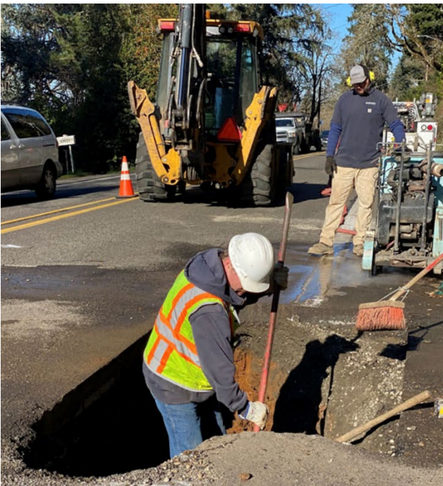
Photo 7: Excavation of leak on Oatfield Road
