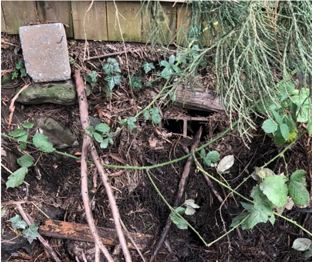
Photo 1: Catch basin clogged with debris
