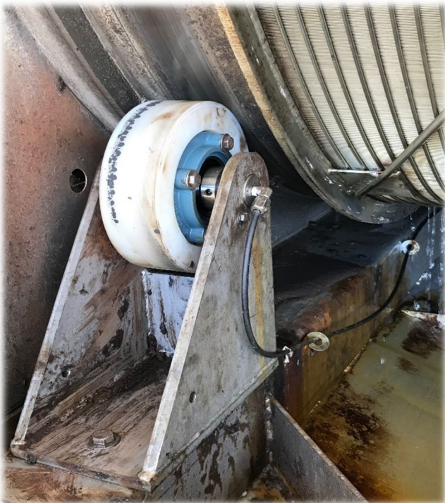
A rebuilt trunnion on the drum screen
