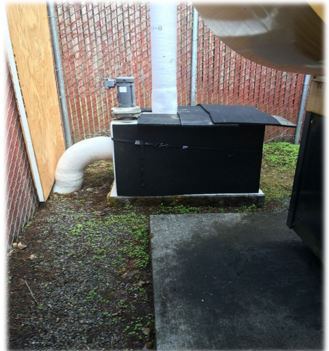
The sound reducing box at Pump Station #2
