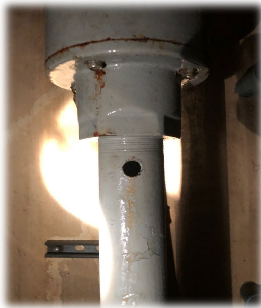
3) Pump Station #6 port in dry well
