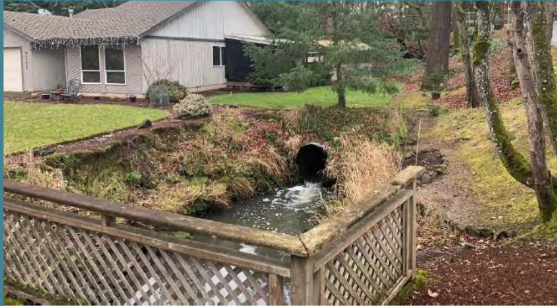
Figure 65. Culvert upstream of SE Walta Vista Rd that is presumed impassable for fish (culvert extends upstream through SE River Road in background of photo, culvert length is an estimated 80 or more meters).
