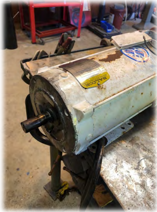
5) Polymer Supply Pump (Dead)
