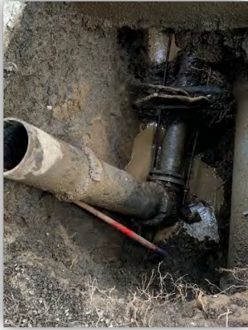
Picture showing broken hydrant after excavation.
