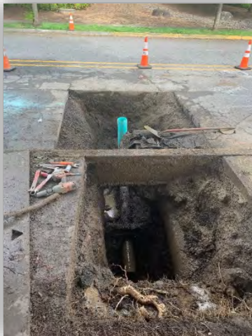
Another Picture showing after the removal of the broken hydrant.
