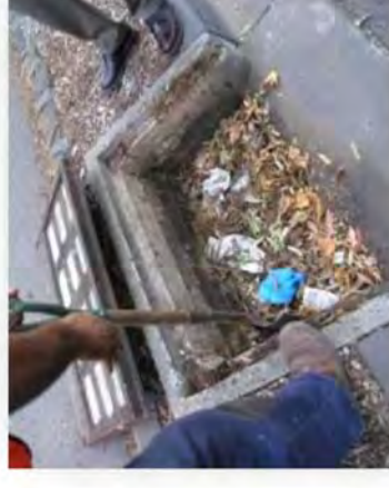
District's SWM maintenance includes catch basin cleaning.
