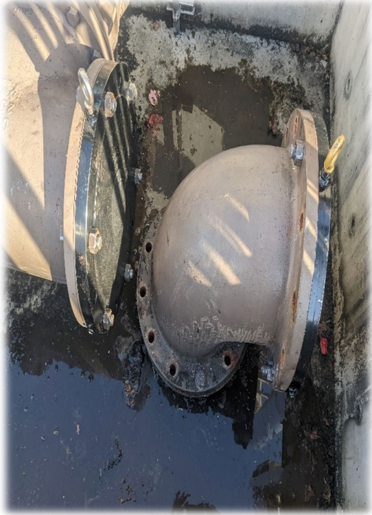
Blind Flange and Cap on Digester Overflow
