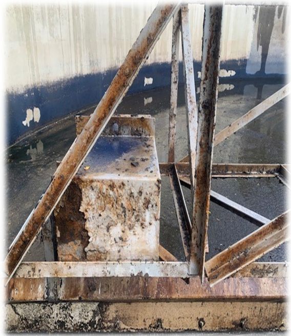
Counterweight on Secondary Clarifier #1
