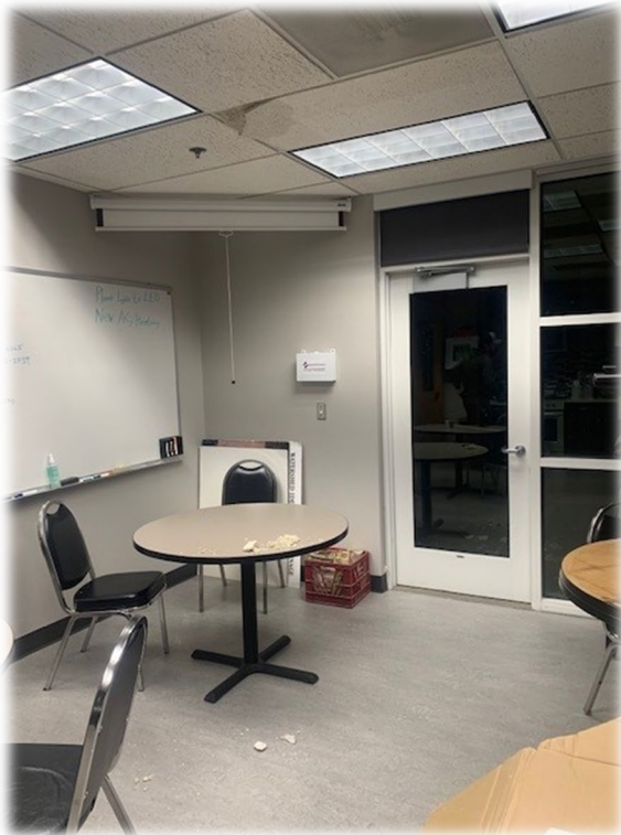
Lunchroom Ceiling Leak
