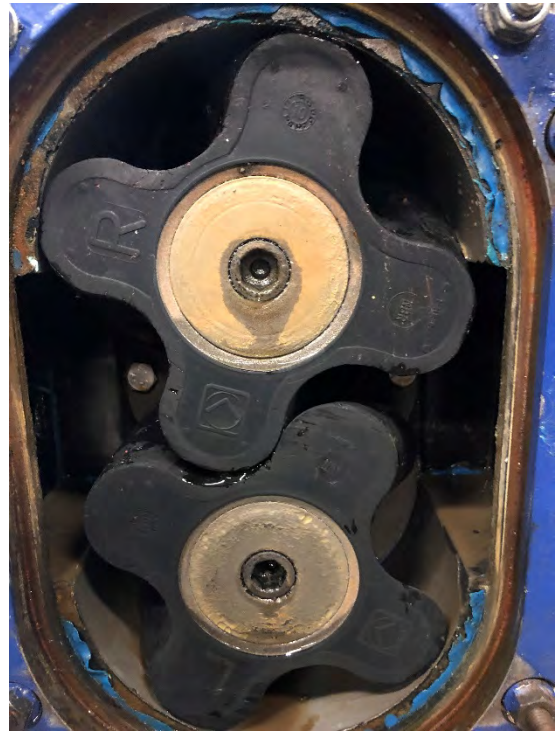
Digested Sludge Pump Lobes Installed
