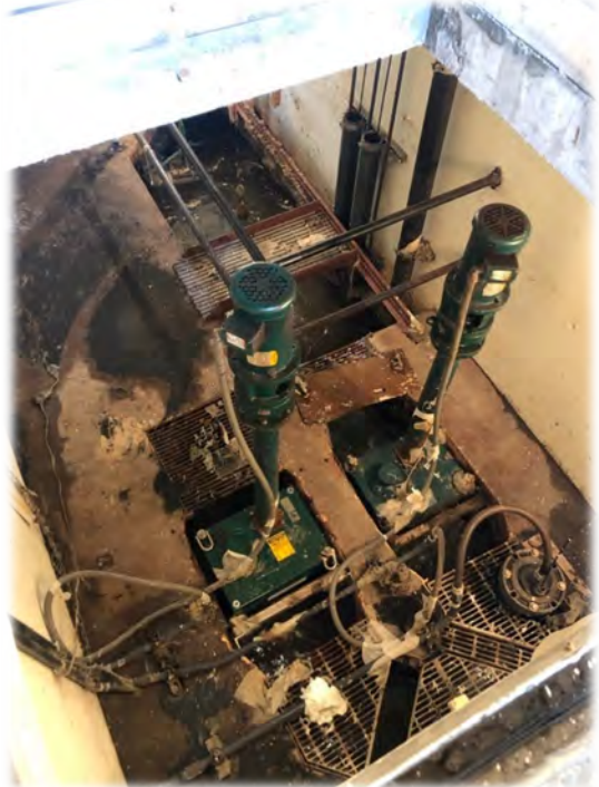
Pump Station #2 Grinders
