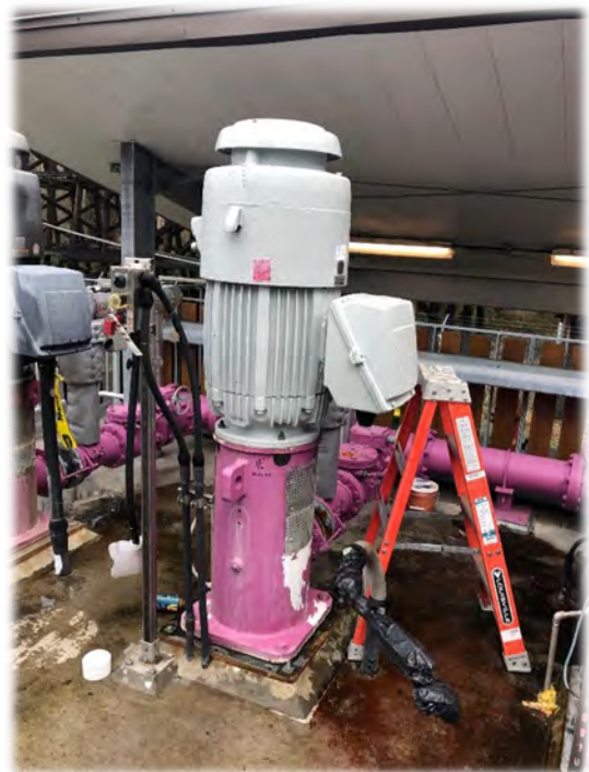
Reuse Water Motor Shellacked
