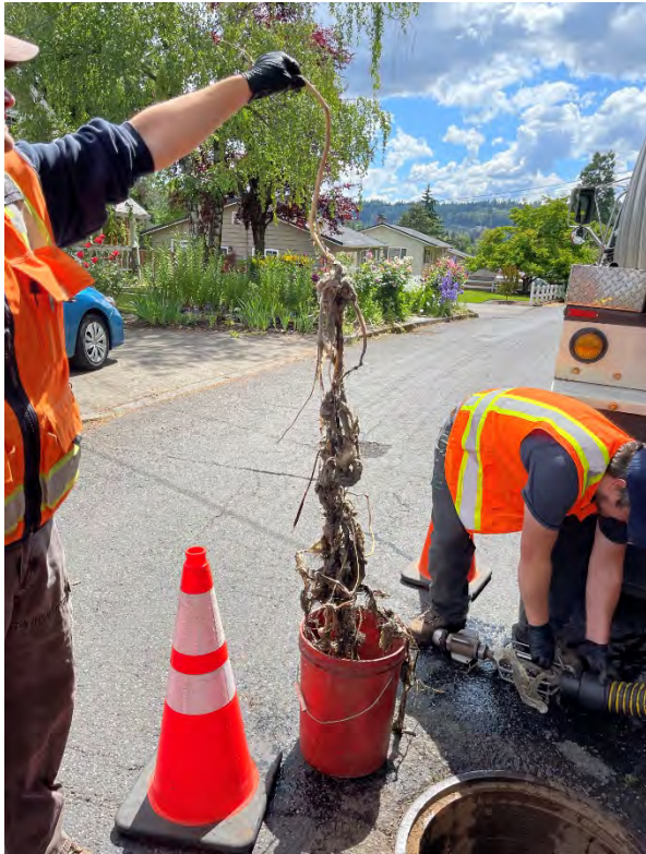
3) Roots Retrieved from Sewer Main
