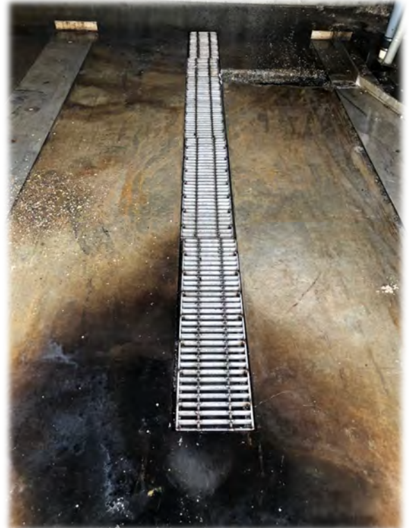
New grating in screenings room
