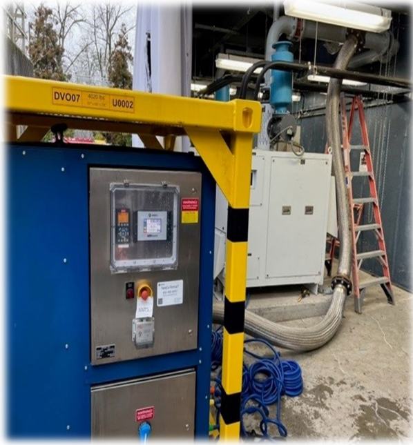
Rental Blower Delivering Air to the Digesters.
