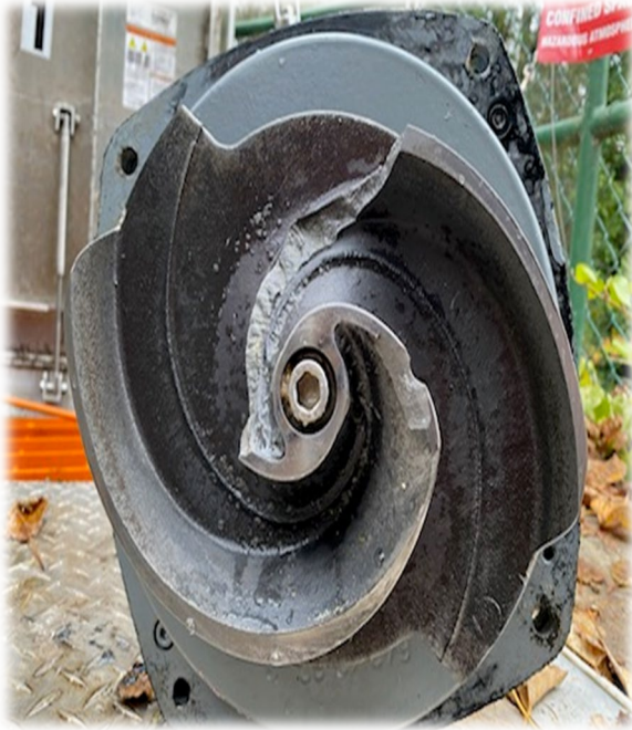
Lift Station #5 damaged impeller.
