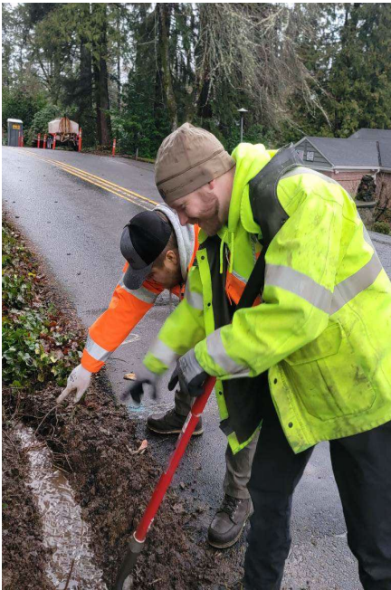
Storm Overflow Diversion
