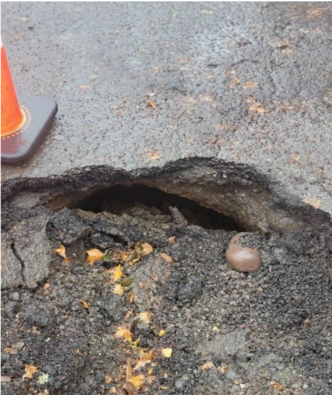
Sink Hole (Redwood Ave)
