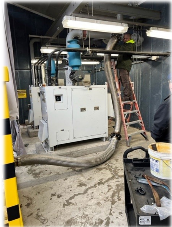
Rental Blower Being Plumbed In.
