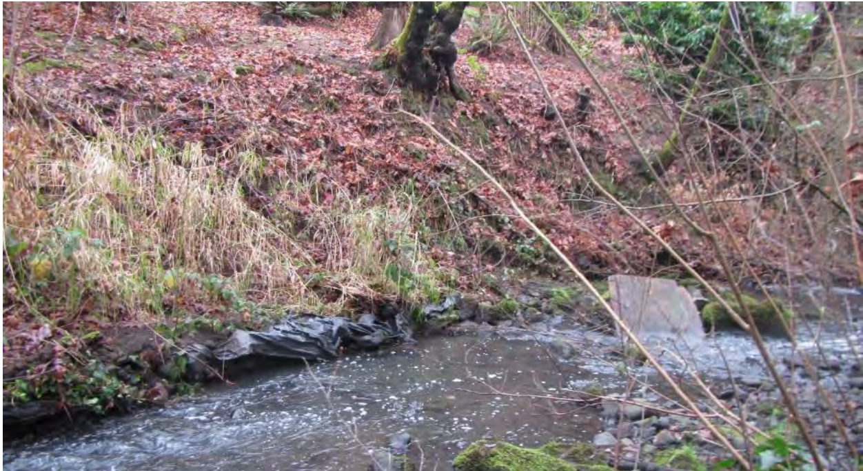
Figure 51. Minor bank erosion (and plastic sheeting along bank, presumably to limit additional erosion) noted along river left bank of Boardman Creek within the reach.
