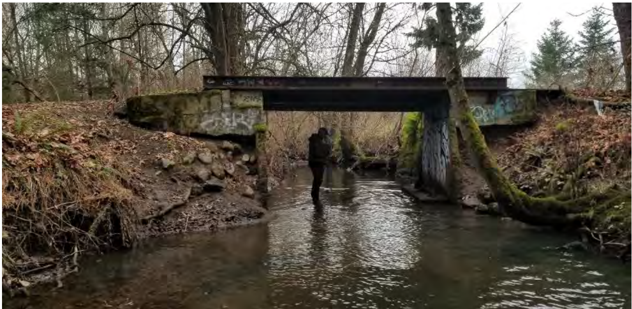
Figure 31. Bridge that crosses over the MSC channel in Reach 3, appearing to constrict flow, near approximately rKm 2.5.
