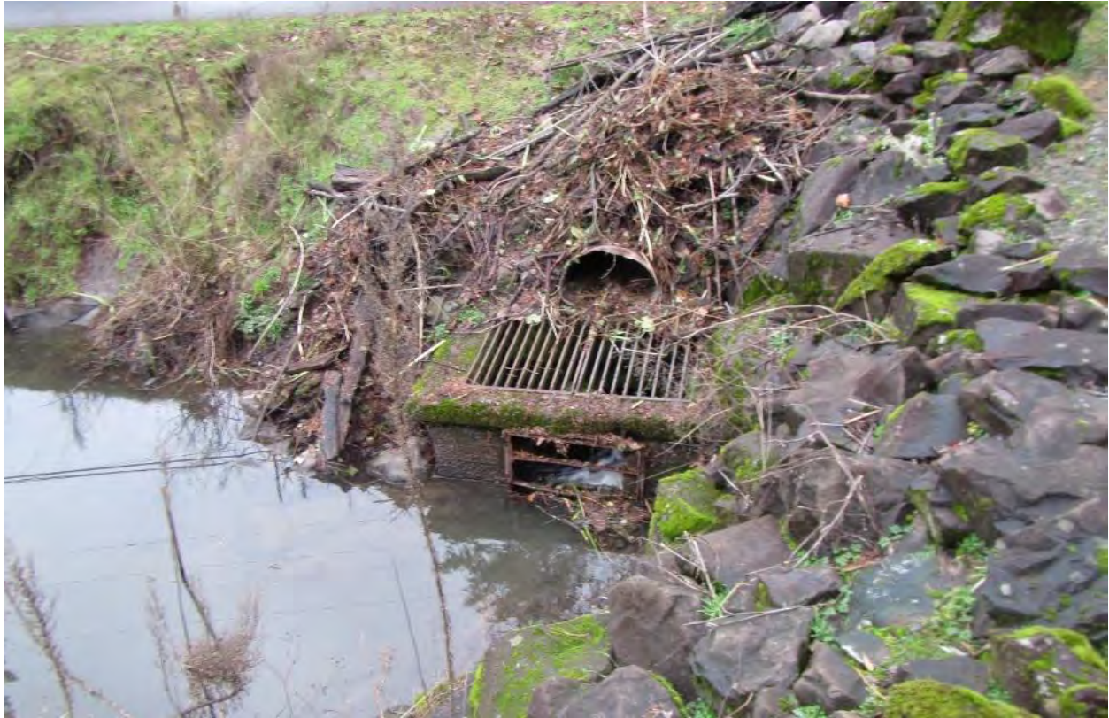
Figure 80. Upstream culvert inlet for SE River Forest Drive crossing, with debris rack and overflow culvert, substantial bank armoring, and debris accumulation. This culvert maintains River Forest Lake water surface levels.
