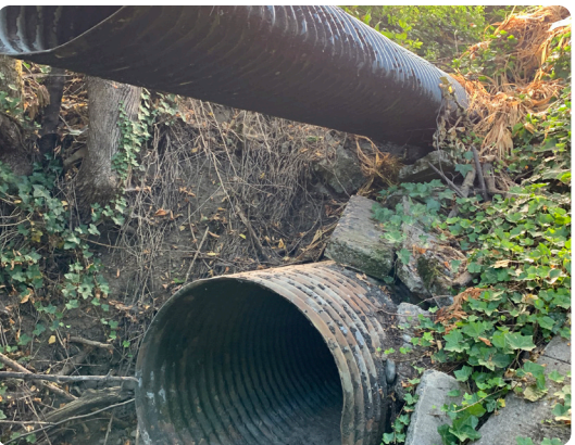
Existing culverts upstream of project area at the River Forest Drive crossing, currently acting as a full barrier to fish passage.
