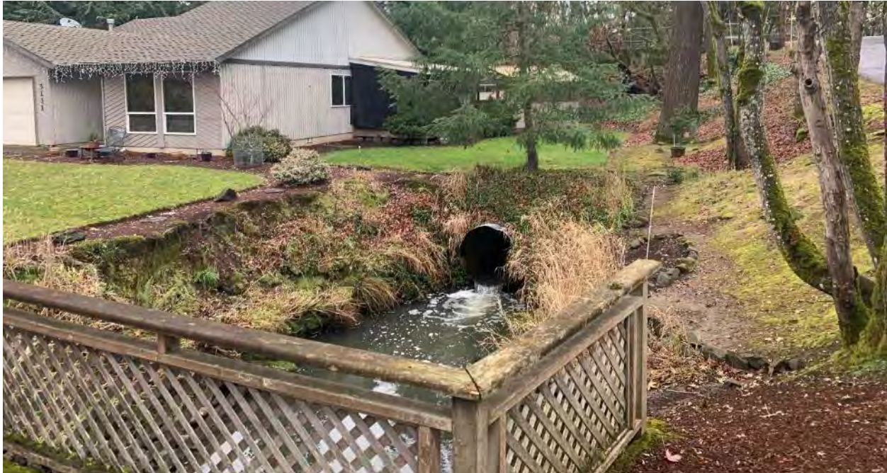
Figure 65. Culvert upstream of SE Walta Vista Rd that is presumed impassable for fish (culvert extends upstream through SE River Road in background of photo, culvert length is an estimated 80 or more meters).
