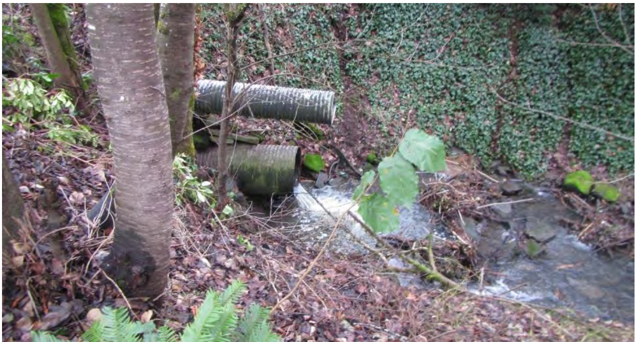
Figure 79. View of outlet of culvert through SE River Forest Drive from river left bank.
