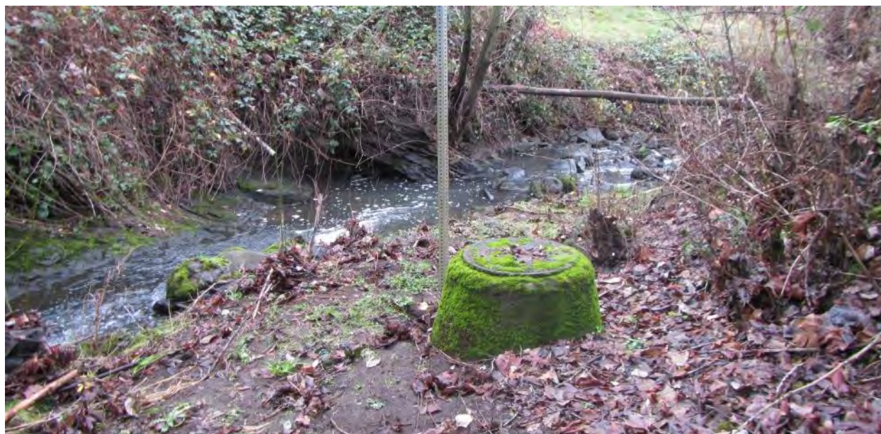
Figure 62. Stormwater manhole located in the river right floodplain near rKm 0.07 of Boardman Creek.
