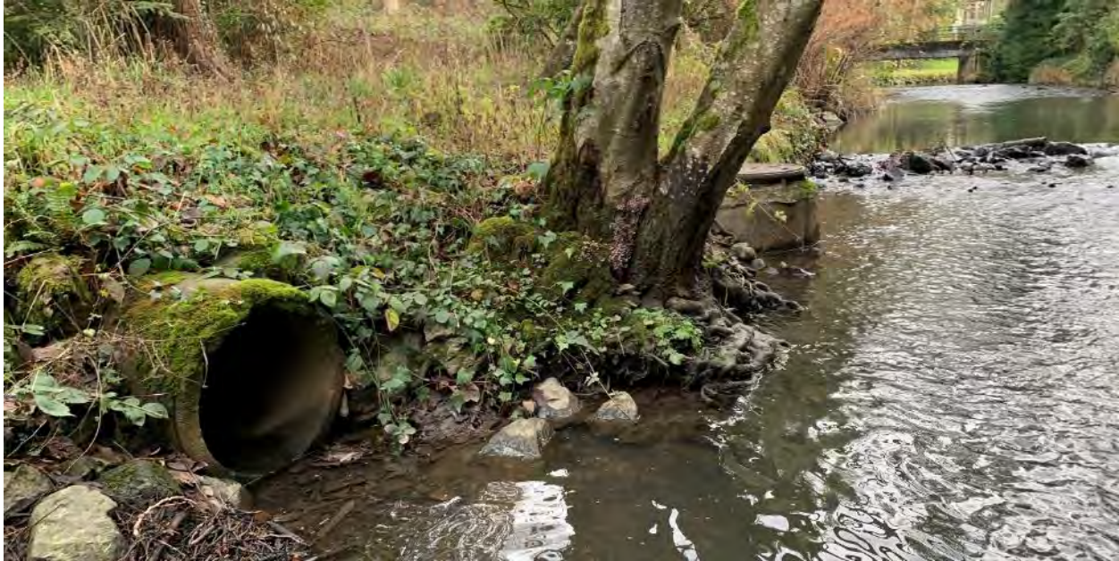
Figure 20. Stormwater outfall (No. 45014) located on the river right bank of Kellogg Creek near rKm 3.06.
