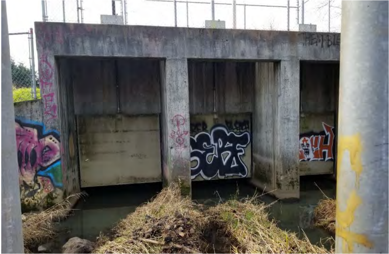
Figure 30. Water control structure gates at rKm 2.2 in MSC Reach 3.
