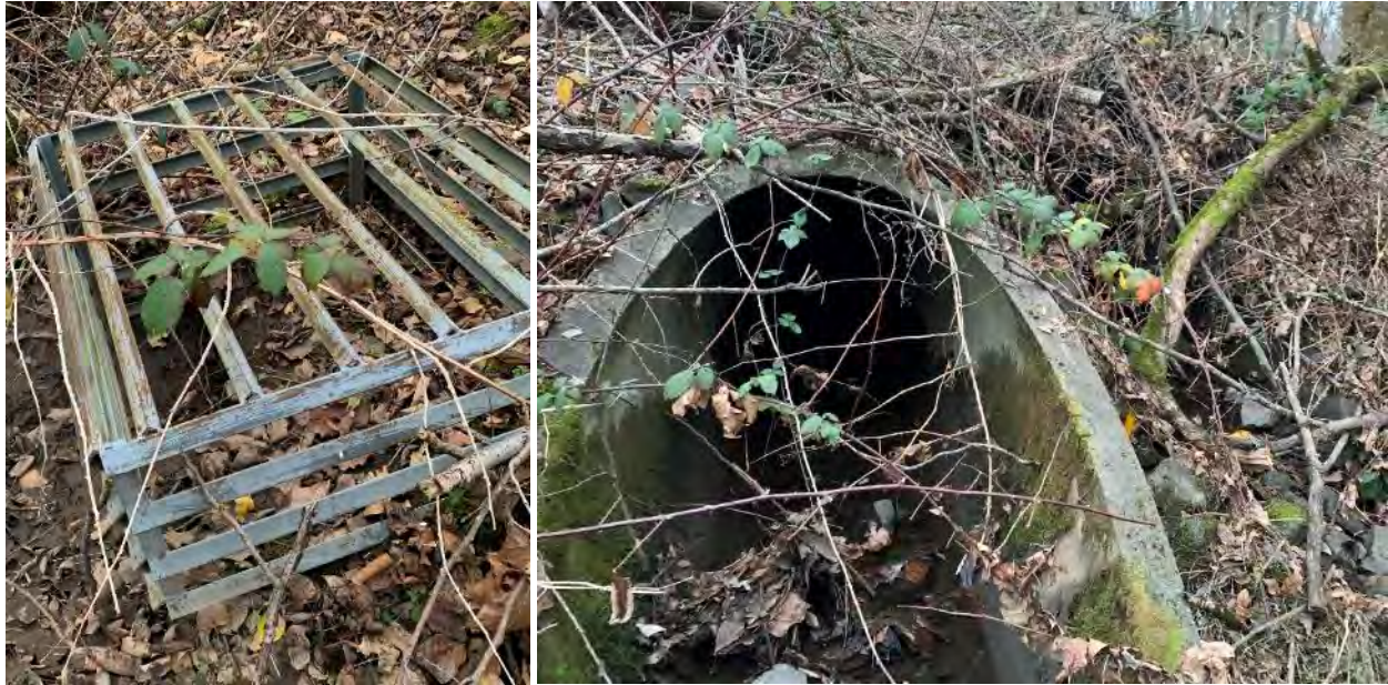
Figure 49. Example stormwater outlet/inlet (?) with a debris rack (left) and two stormwater outfall culverts in MSC Reach 5.
