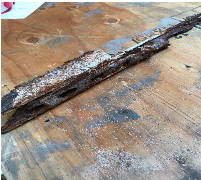
Photo 6 Corroded Support Bar
