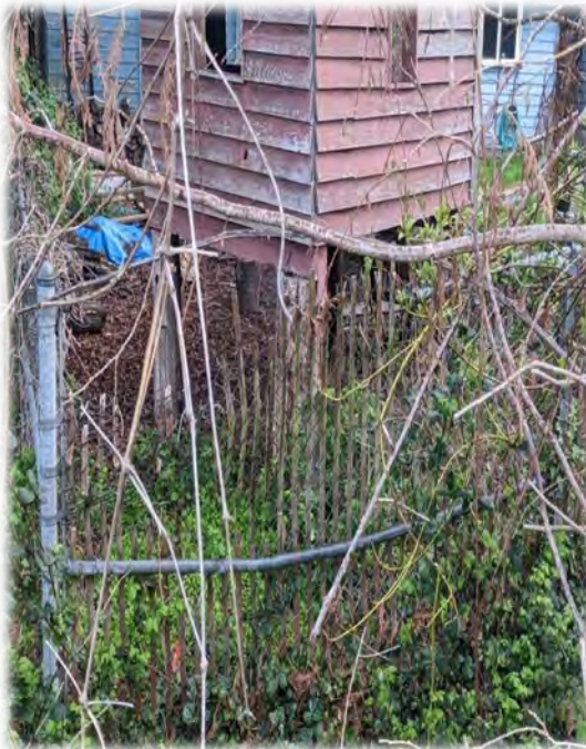
Fence before repair.
