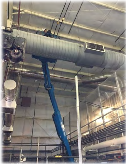
Changing light bulbs in the solids building.
