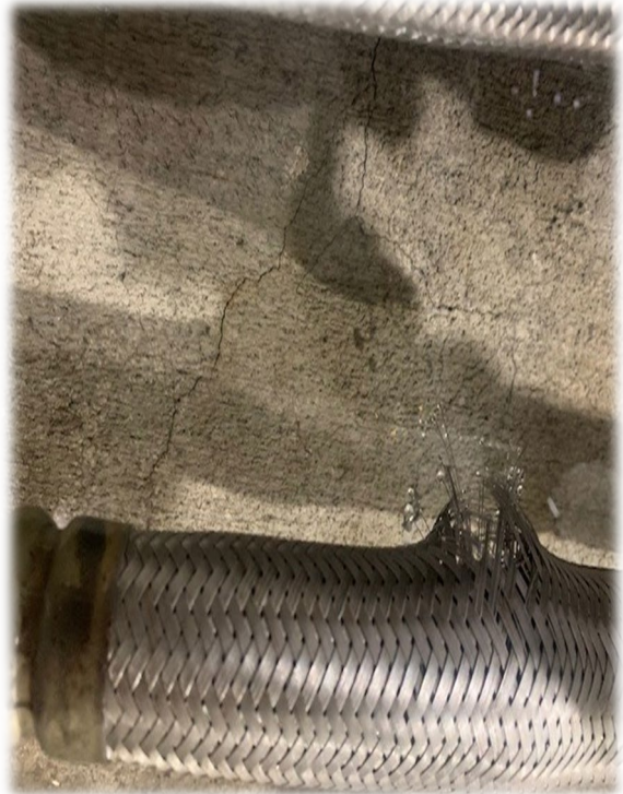
Braided Water Line That Broke.
