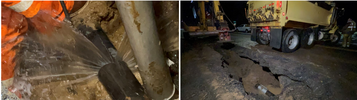
SE River Rd Main Break
